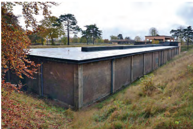
The roof of the central Non-nuclear Component blockhouse showing the reinforced concrete framed construction, the roof and its central air conditioning duct, and at the far end the raised lifting gantry
